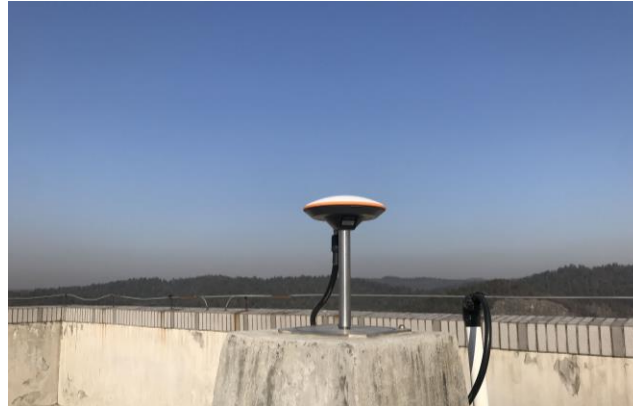
Fig. 5 Monitoring equipment No. 1 in an ideal environment
