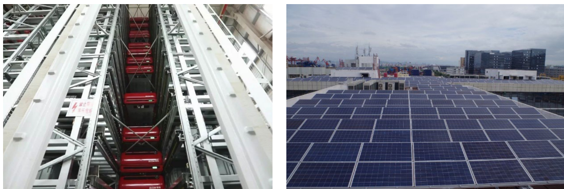
Figure 1: SBS/RS and rooftop PV (Source: left: Cao (2020); right: Xiamen Container Terminal Group (2021))
