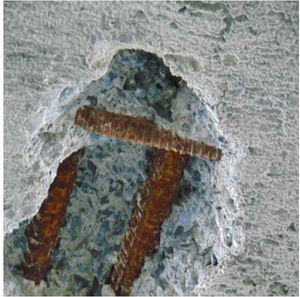
(b) Spalling- Image "B"
