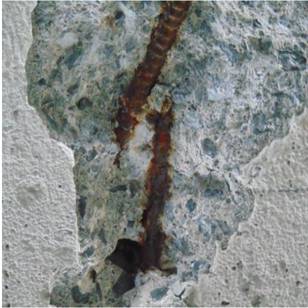
(a) Spalling- Image "A"
