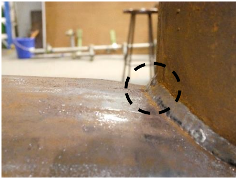
a) Plastic deformation at crown point
