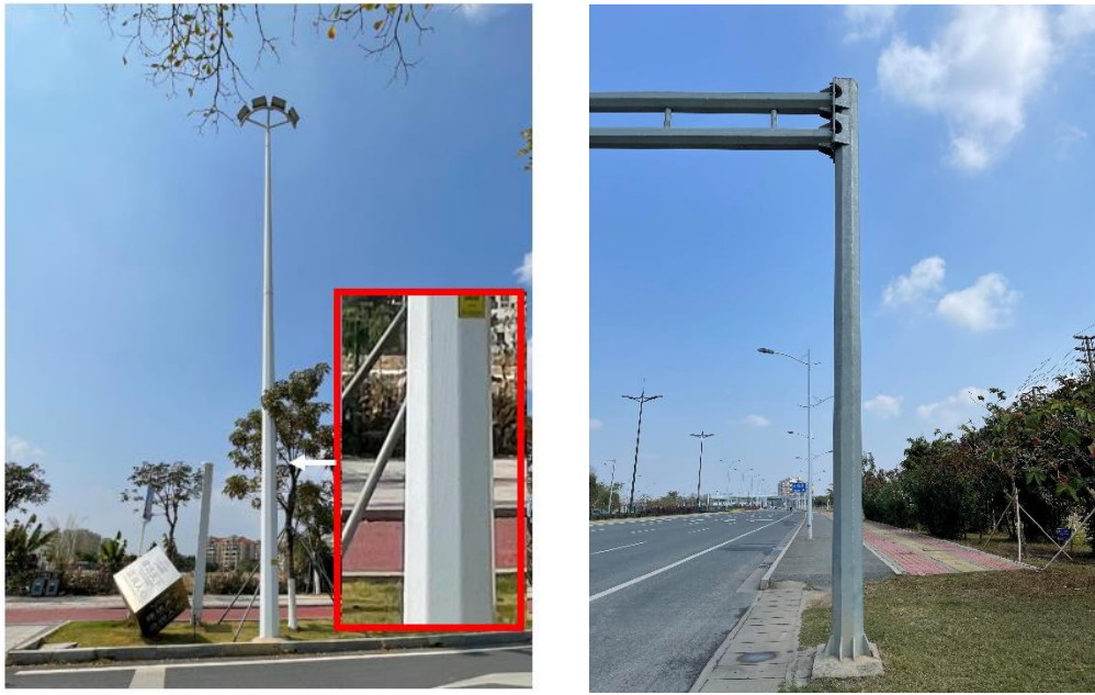
(a) Fig. 1. Application of the octagonal sections in civil engineering structures (a) Octagonal section lighting column (Zhuhai, China) (b) Octagonal section steel columns (Shenzhen, China).
