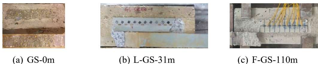
Fig. 12. The failure mode of GSB.
