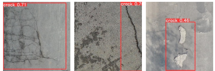
Fig. 19. Crack detection performance on asphalt pavement scene.
