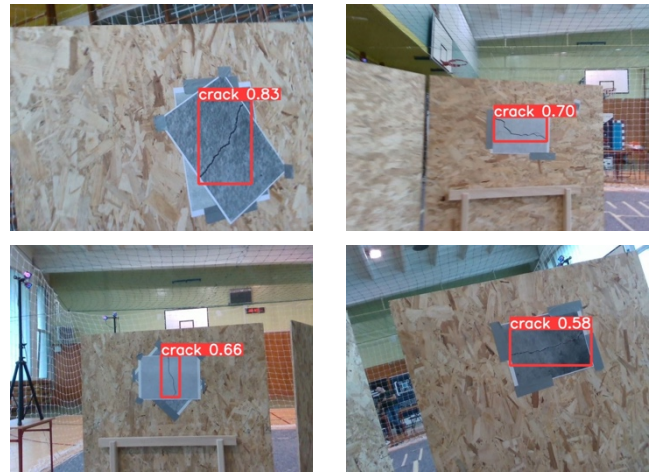
Fig. 18. Crack detection tests with wooden boards background.
