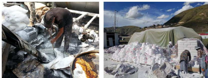
Figure 14 The incorporation of nanomaterials into asphalt binder or asphalt mixture (taken by the authors from the field)
