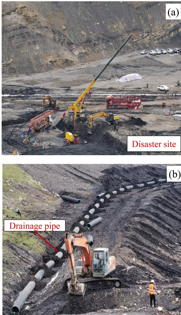
Figure 6. Drainage facilities at the rescue site: (a) the disaster site and (b) drainage pipe (recreated based on Qi 2021).
