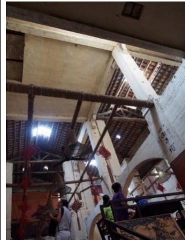
Fig. 2.25 The typical structure system of arcade buildings on West Embankment Street, Chikan Ancient Village, Kaiping. 33
