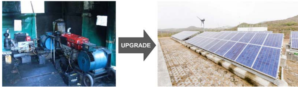
Figure 1 - Diesel generator used to power Town Island before system upgrade (left) [22] and Town Island Microgrid (right) [23]
