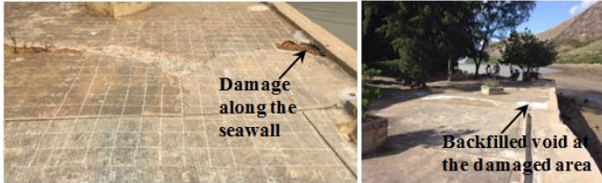
Figure 9 GPR grid pattern at Tai O and void visible from the ground (left) and void after backfill
