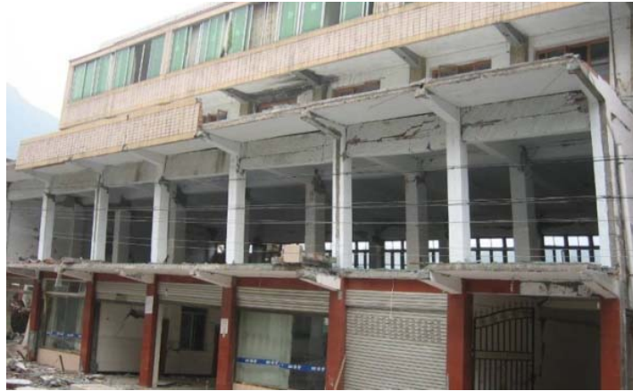
Figure 2. Failure at column ends
