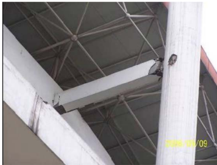
Figure 3. Failure at beam ends
