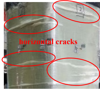
Fig. 5 Horizontal cracks on a typical specimen
