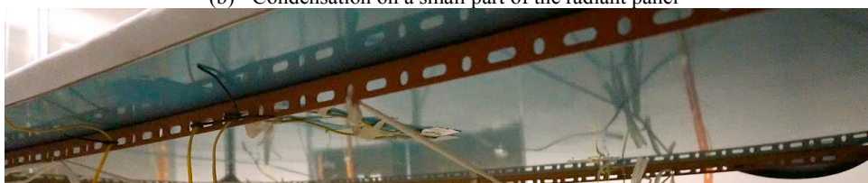
(c) No condensation on the radiant panel
