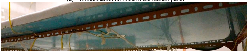
(b) Condensation on a small part of the radiant panel
