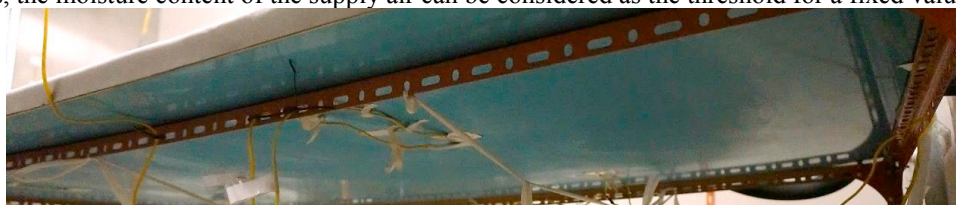
(a) Condensation on most of the radiant panel
