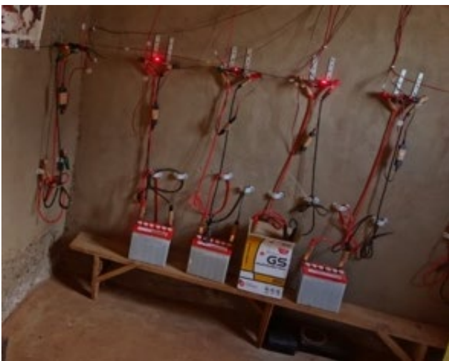
Fig. 2. A charging station being installed (up), and the interior charging room (down). The panels are permanently attached to six controllers. Community members bring their depleted batteries and plug them in for charging.
